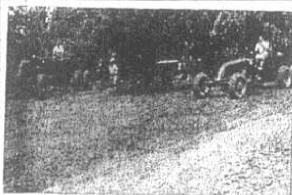
Road graders and bulldozers were on the job Sunday, clearing a wooded area on the Community Center playground for another St. Matthews Little League ball diamond. The equipment, two dozers and two graders, was donated by the Williams Tractor Co. They are being handled by Clint and John Carber, and Clint's son, Dean, who donated their time. Also pictured is John Gambill, chairman of the project. The new diamond should be ready to go in a couple of weeks, said Mr. Gambill. Either a third Little League will be created or the minor league will play this year. But next year, there will definitely be a third major league, he said. The new diamond is directly behind the present Little League diamond.
